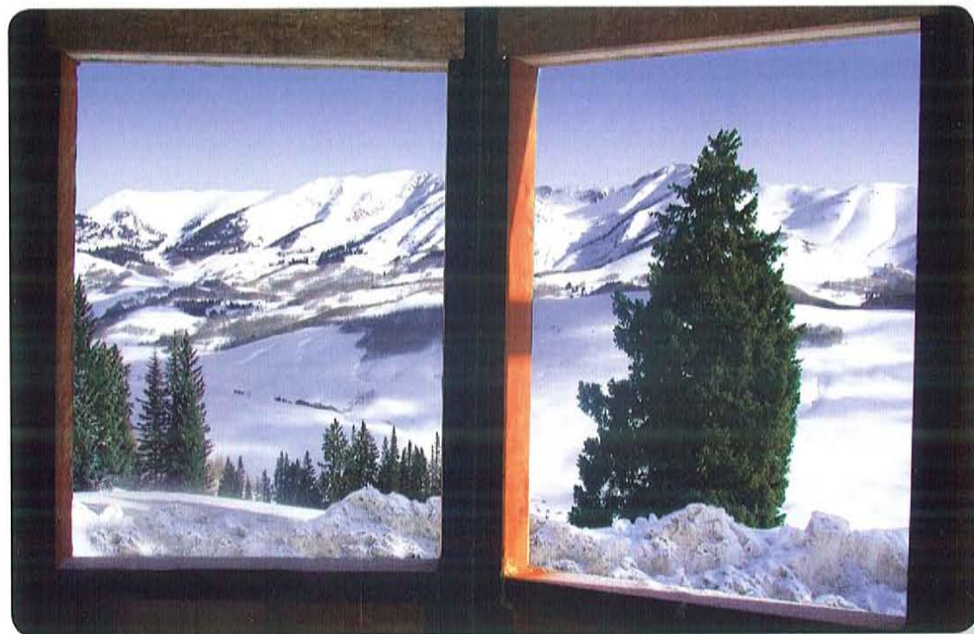
ABOVE: Spectacular views, of the Elk Mountain range, from the Master Bath window of the Tipple House (under construction until fall 2009). Note the insulated headers and LVL framing.
